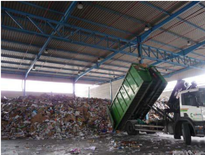
Unloading and storage of loose recovered paper in an enclosed facility with a roof
