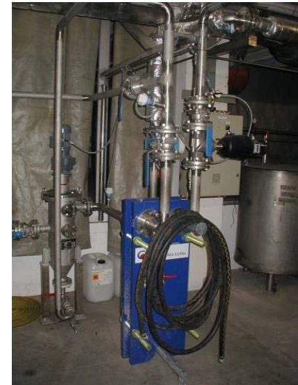
Heat exchanger with filter
