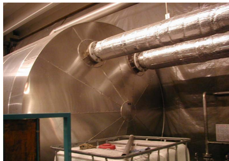
Proper heat-insulation of pipes
